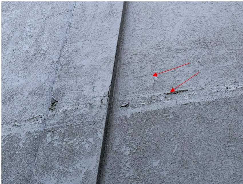
Figure 6: Cracking at east (lakeside) wall
