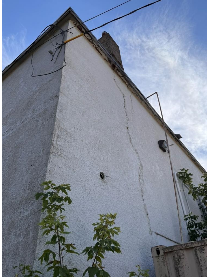
Figure 4: Vertical crack at back wall of building
