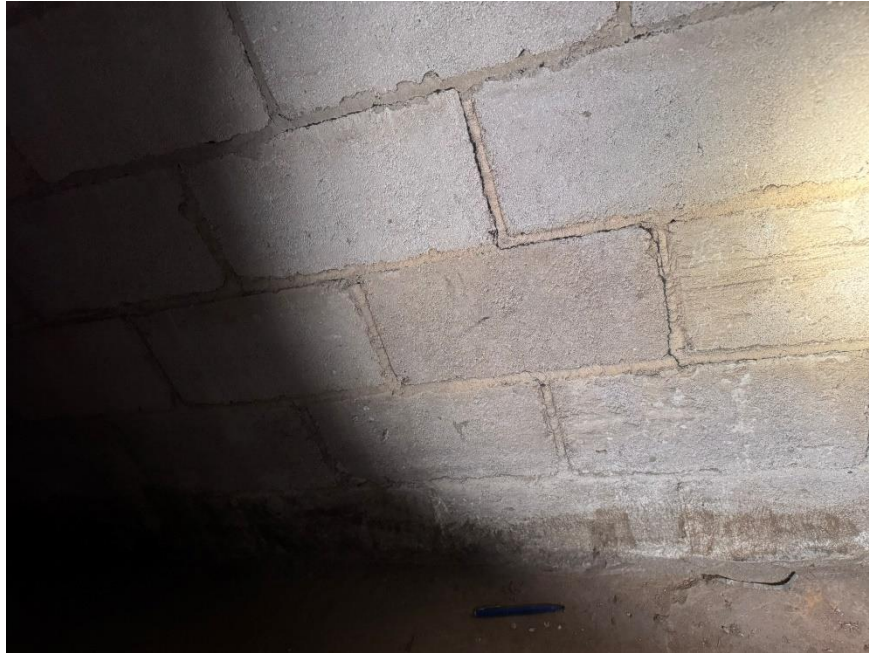
Figure 5: Basement wall cracking adjacent to east wall (looking south)
